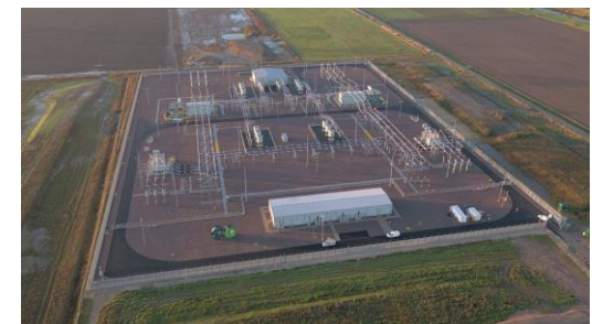
Wind Farm Substation Ariel Views
