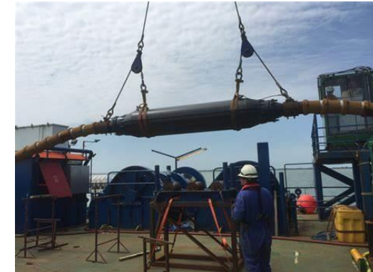
Cable Joint on Vessel
